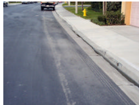
Stain from water in the gutter.
