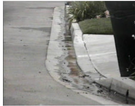
Pavement stain waiting to happen!
