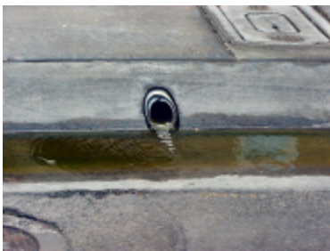
Backyard water draining to street.
